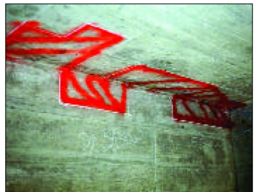
Delaminated concrete is marked. Courtesy of Great Western Corporation
