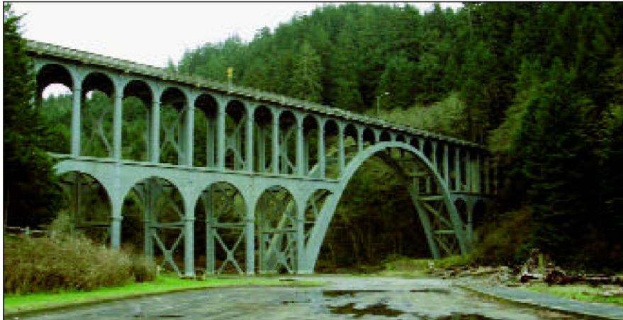
Cape Creek Bridge, the first of Oregon's historic bridges to be metalized (1991) Courtesy of the Oregon DOT
