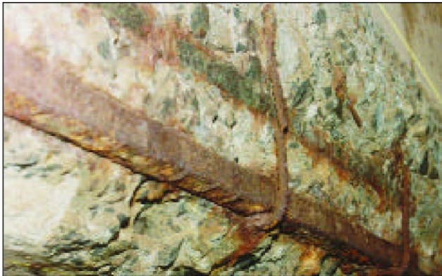
Typical coastal bridge damage Courtesy of the Oregon DOT
